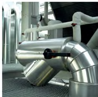
Air conditioning application
